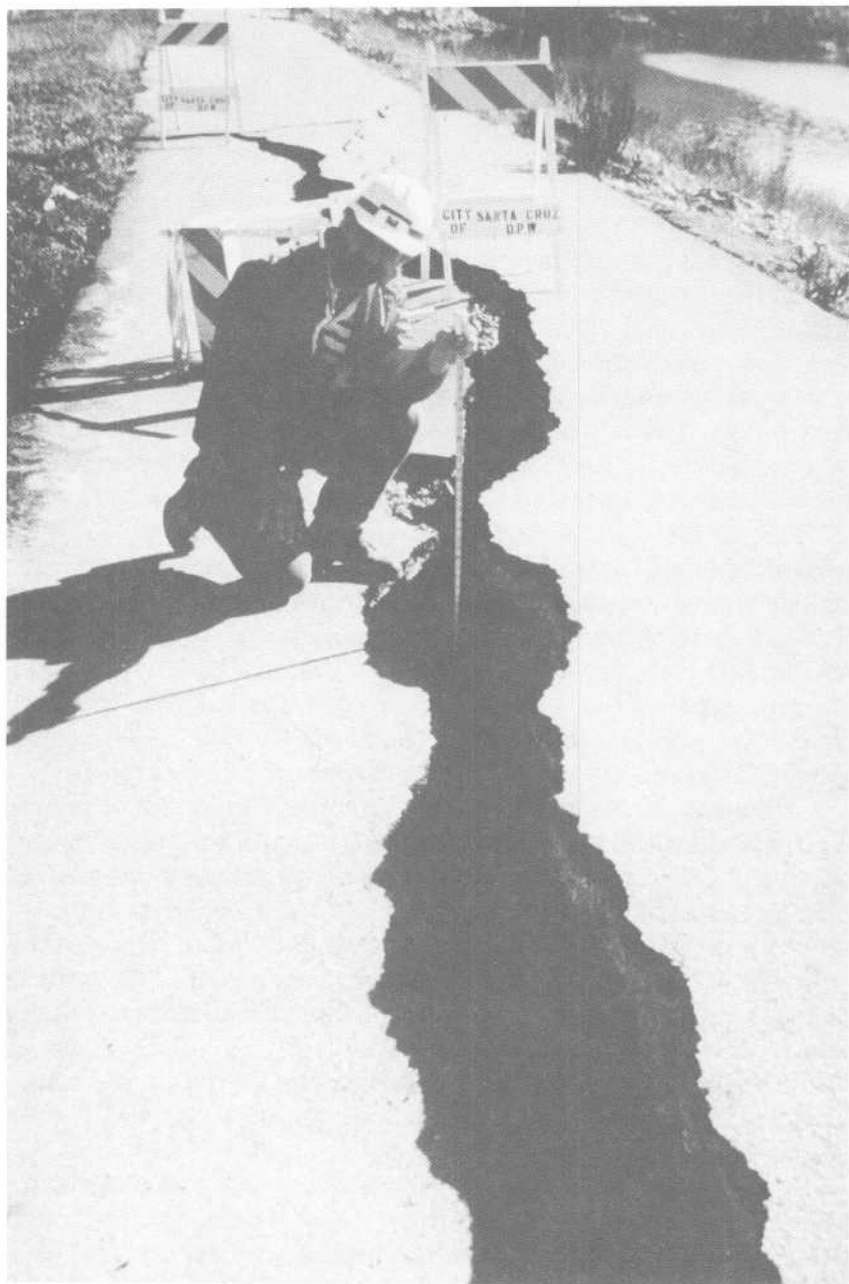
A Corps inspector measures a fracture in the Pajaro River levee.
