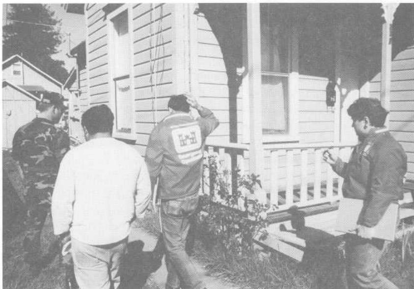
A Corps of Engineers team investigates the damage to a home in Watsonville, California.
