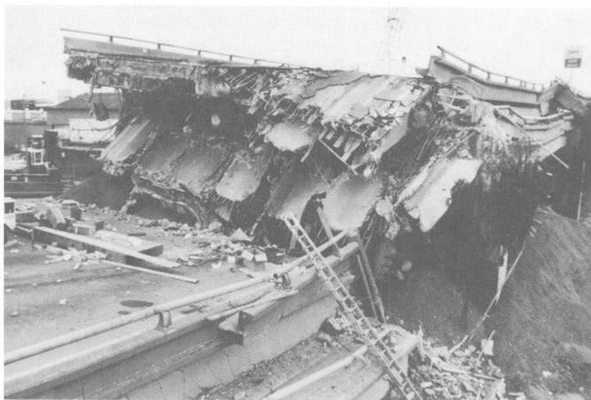
A collapsed section of the two-tiered I-880 in Oakland, California.
