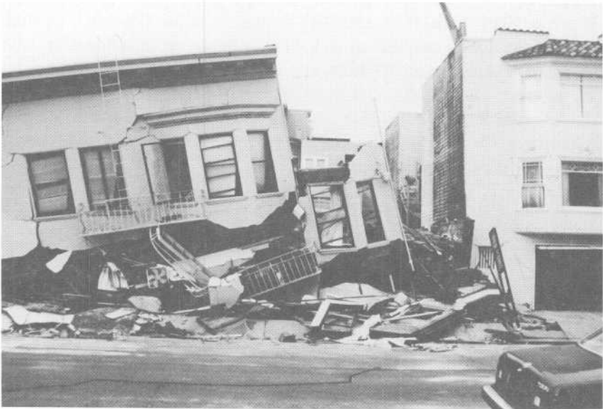
The most heavily damaged section of San Francisco was the Marina district where four people died.
