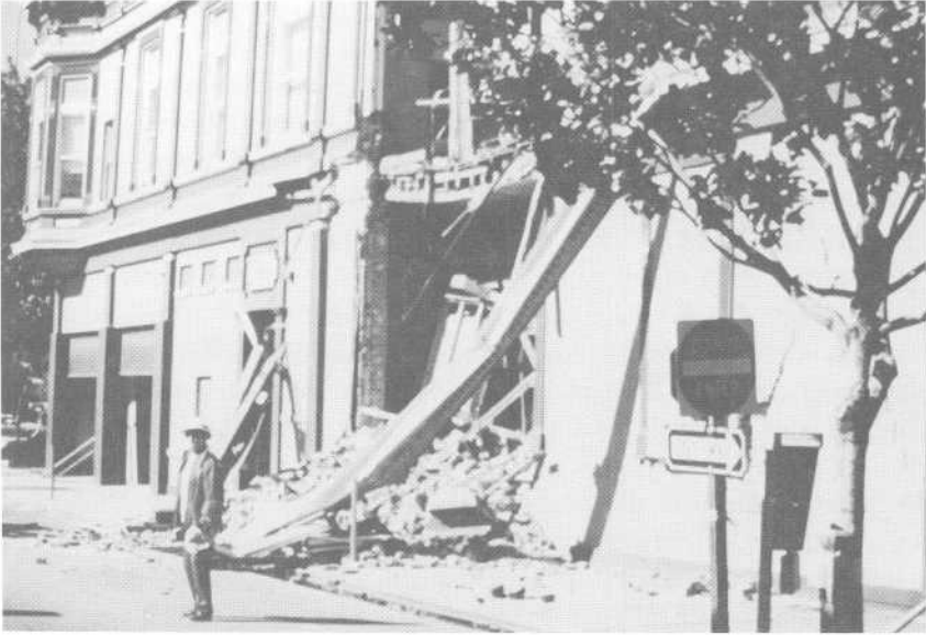
A Corps of Engineers inspector surveys wreckage at the Pacific Garden Mall in Santa Cruz, California.
