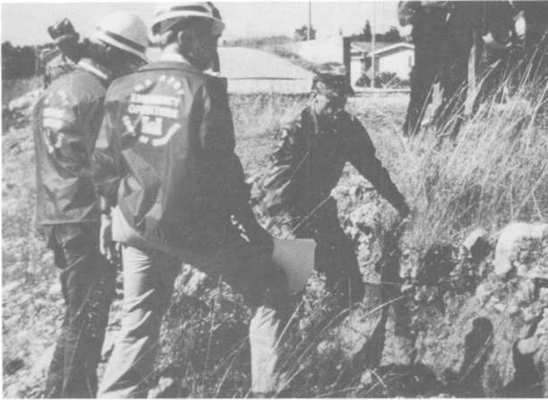
Chief of Engineers LTG Henry Hatch and Corps inspectors examine the San Lorenzo River levee damage.
